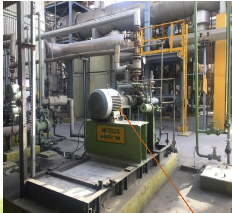
Motor Driven LTS out separator condensate Pump (MP-3323B)
