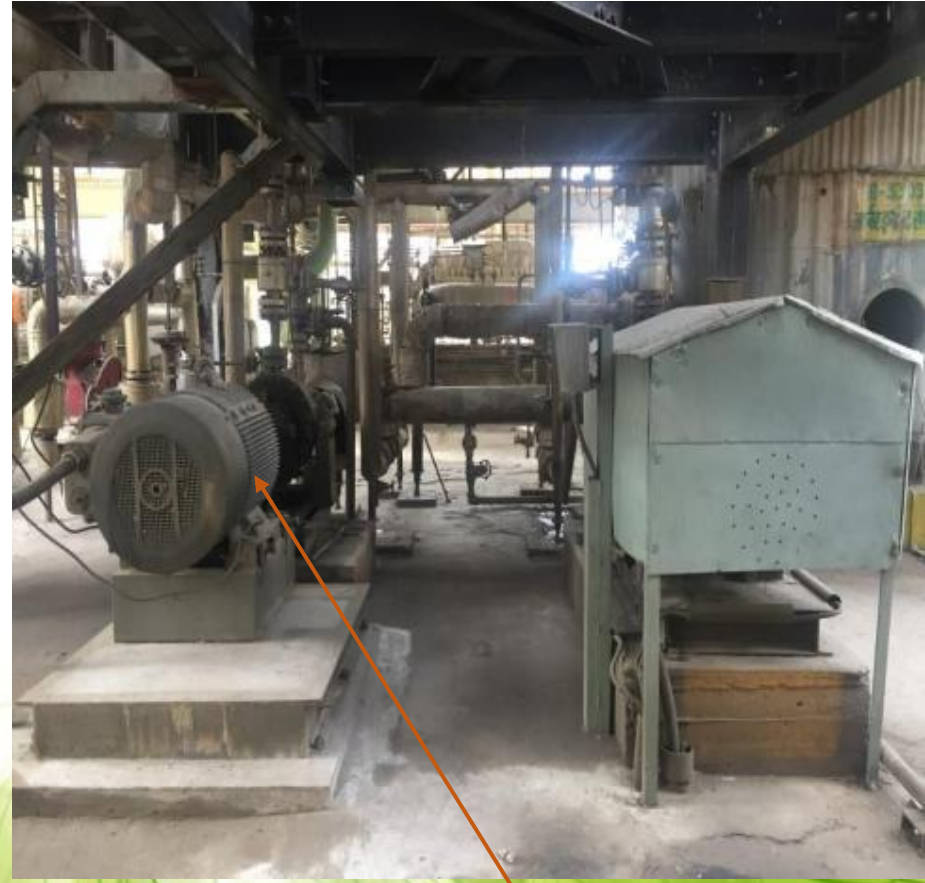
Motor Driven Bulk Absorber Inlet Separator condensate Pump (MP-3323B)
